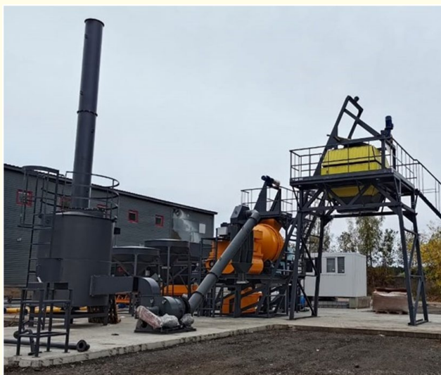
Figure 14: Commissioning works at the installation for the production of foam concrete mixtures in MADI.
