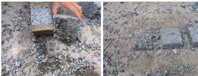
Figure 4: Adhesion of bonding material treatment of polymer-painted cement interface. (Cement concrete base course damage in the left, and surface course damage in the right)
